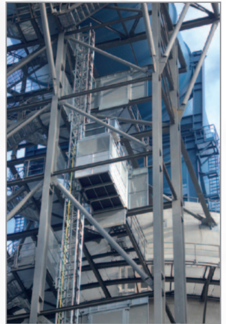
Permanent installation in a power plant
