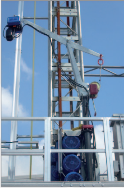
Assembly winch on the cabin roof
